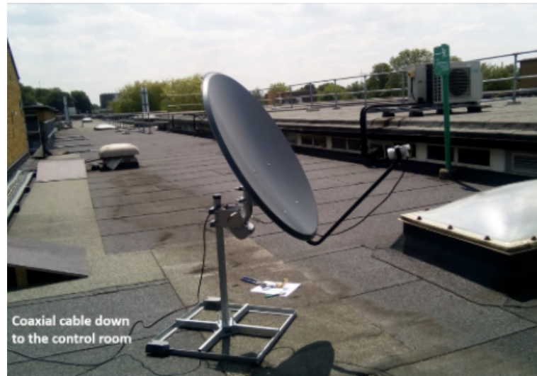
Figure 5.1: Shows the setup of the one- meter off the shelf radio telescope up the roof of the STRI building at the University of Hertfordshire
