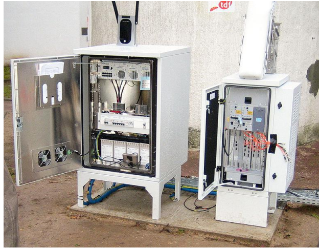
Figure 3.1.2.1: Base Station: Wireless Base Station Equipped with a Sector Antenna and Wireless Modem (Application Note, 2006)
