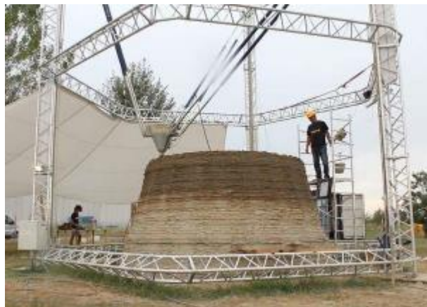
Figure 9 WASP-Big Delta project. Full size 12m building out of mud and clay (WASP-BigDelta, 2012).
