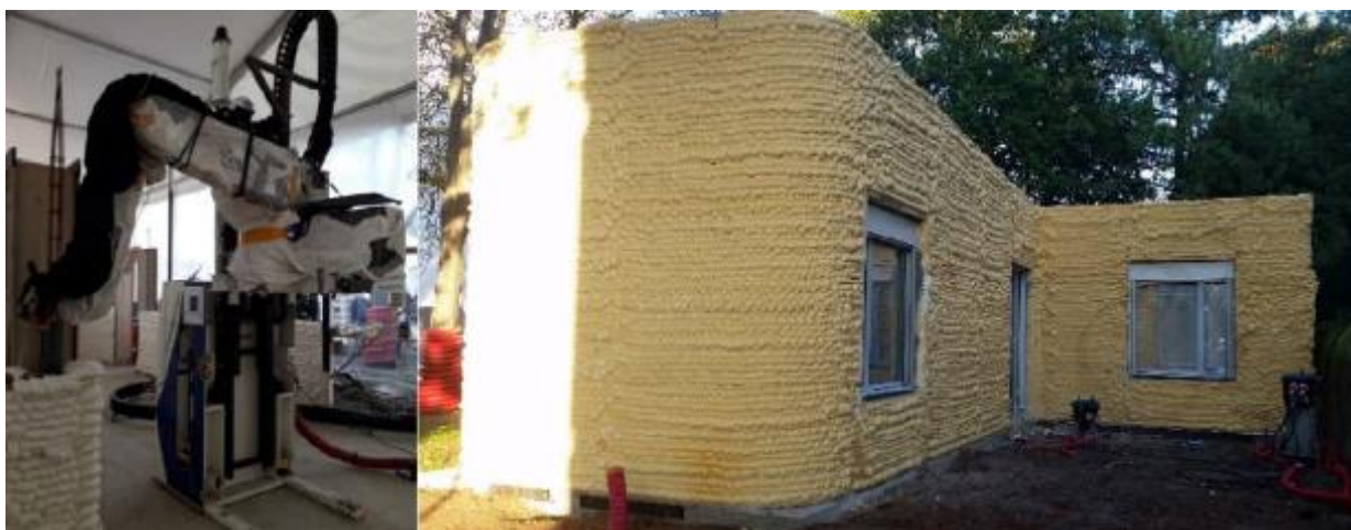
Figure 7 Application of 3D polyurethane printing foam (left) for construction of a dwelling house by using the Batiprint3D technique. The 95 sq. meters printed house is located in Nantes (France) and took only 54 hours to build (right) (Furet et al., 2019).
