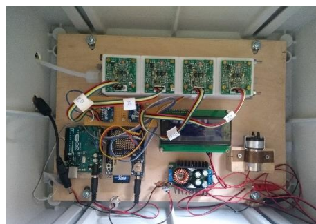
Fig.1 Sensor platform with electronics
